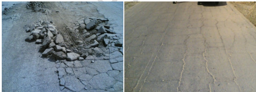
Fig.6: Condition of Dikwa-Gomboru Road.
