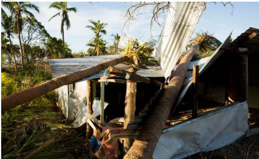
Fig. 3: A community collection center being damaged by the cyclone PAM
