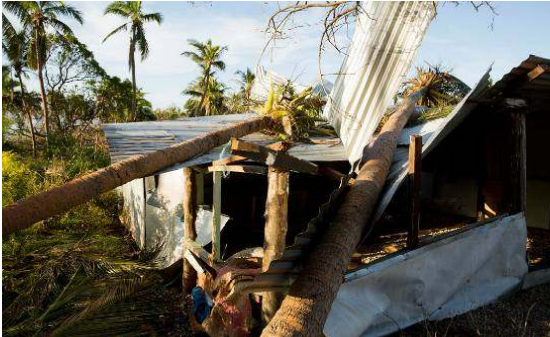
208 209 Fig. 3: A community collection center being damaged by the cyclone PAM 210
