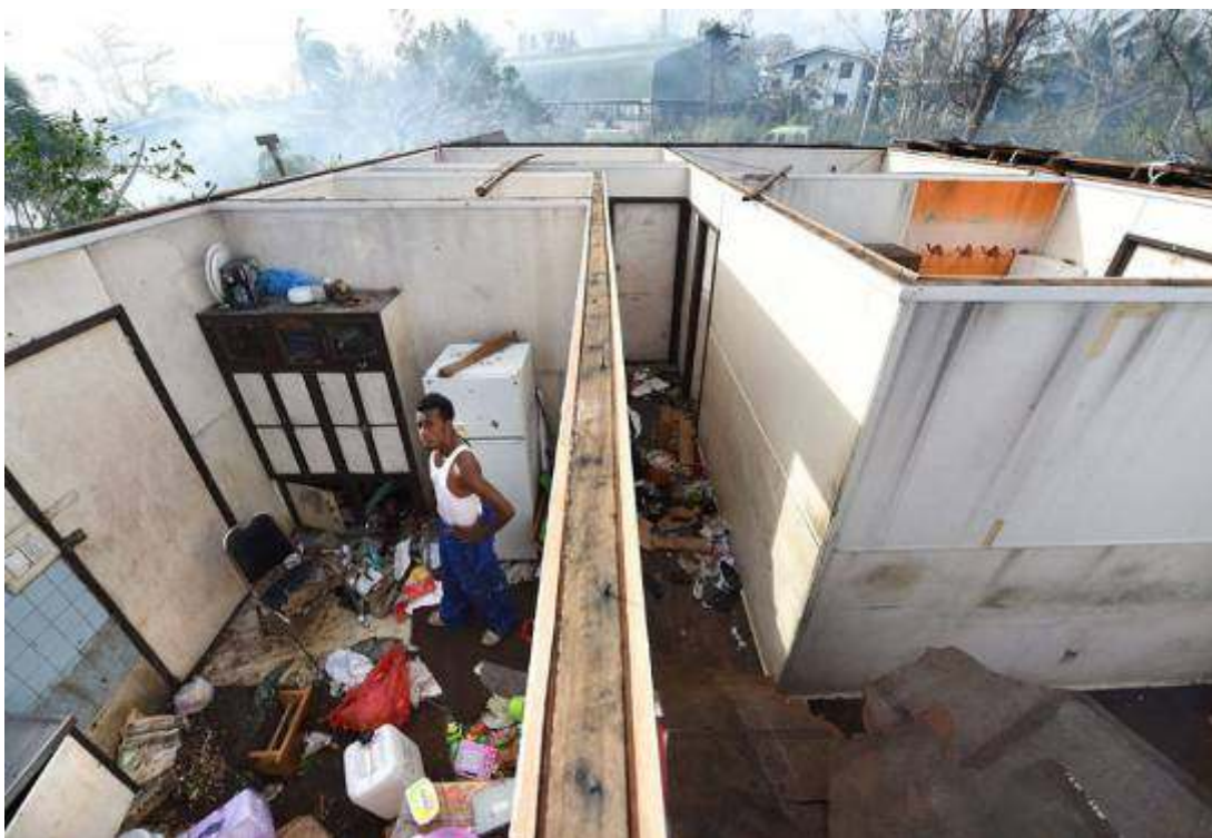
Fig. 4: Roof for the collection of rainwater being blown by the cyclone PAM
